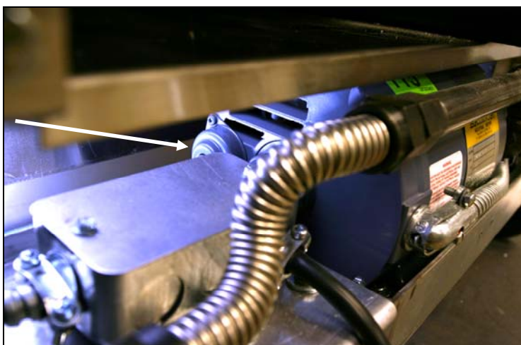
Filter Pump Reset Switch (Arrow)
